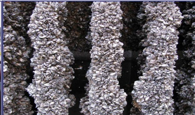
Quagga mussels on Hoover Dam trash rack. Source: USBR.
