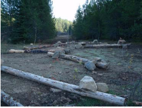
Scour erosion treatment and protection for new riparian tree and shrub plantings.
