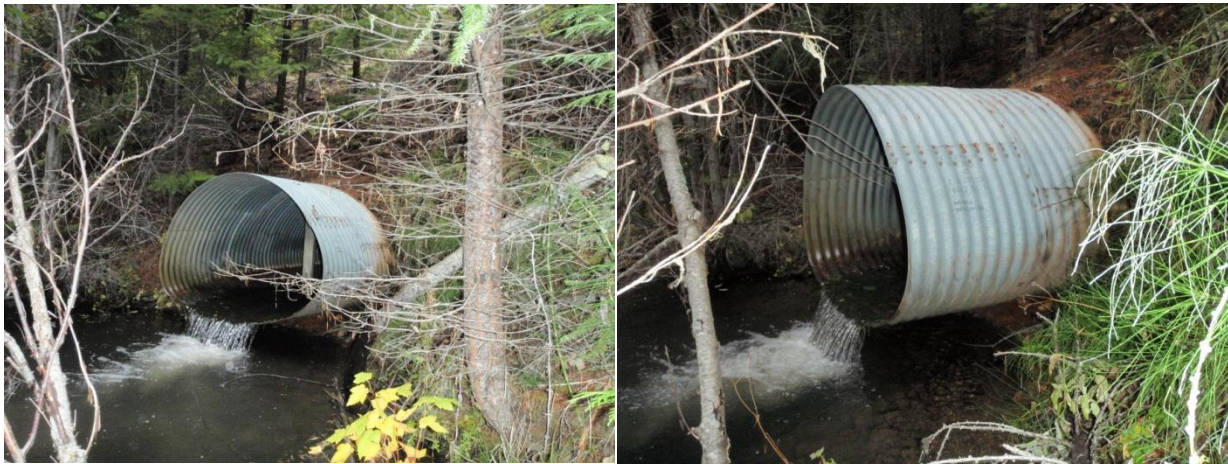
Figure 4. A corrugated culvert on Indian Creek connected to a road prism to be removed to reconnect the stream to its natural floodplain in the Beaver Creek watershed, lower Deschutes River, Oregon.
