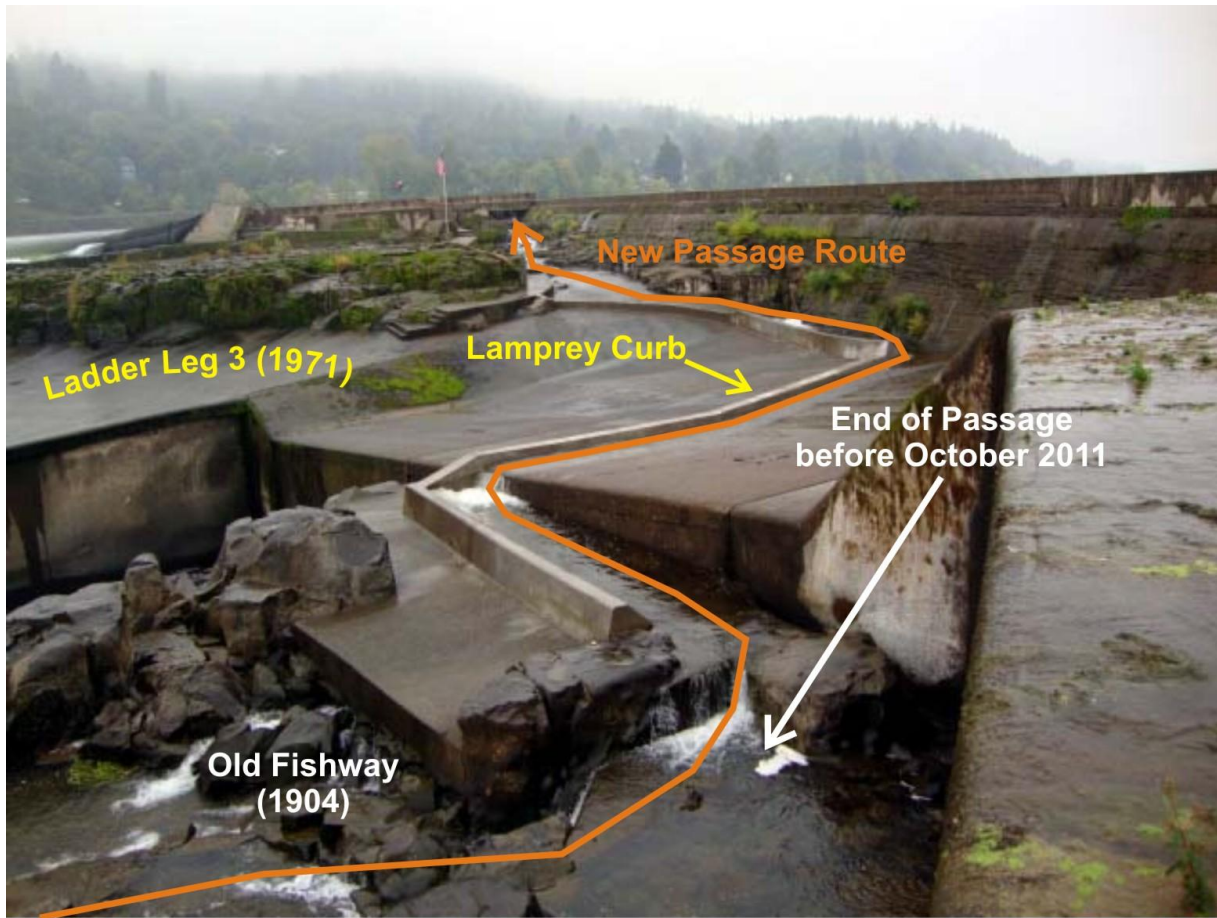
Figure 13. Passage improvements to restore lamprey passage through the old fishway, October 2011 (picture courtesy of Tim Shibahara, PGE).
