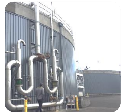
Columbia Boulevard Digesters 34
