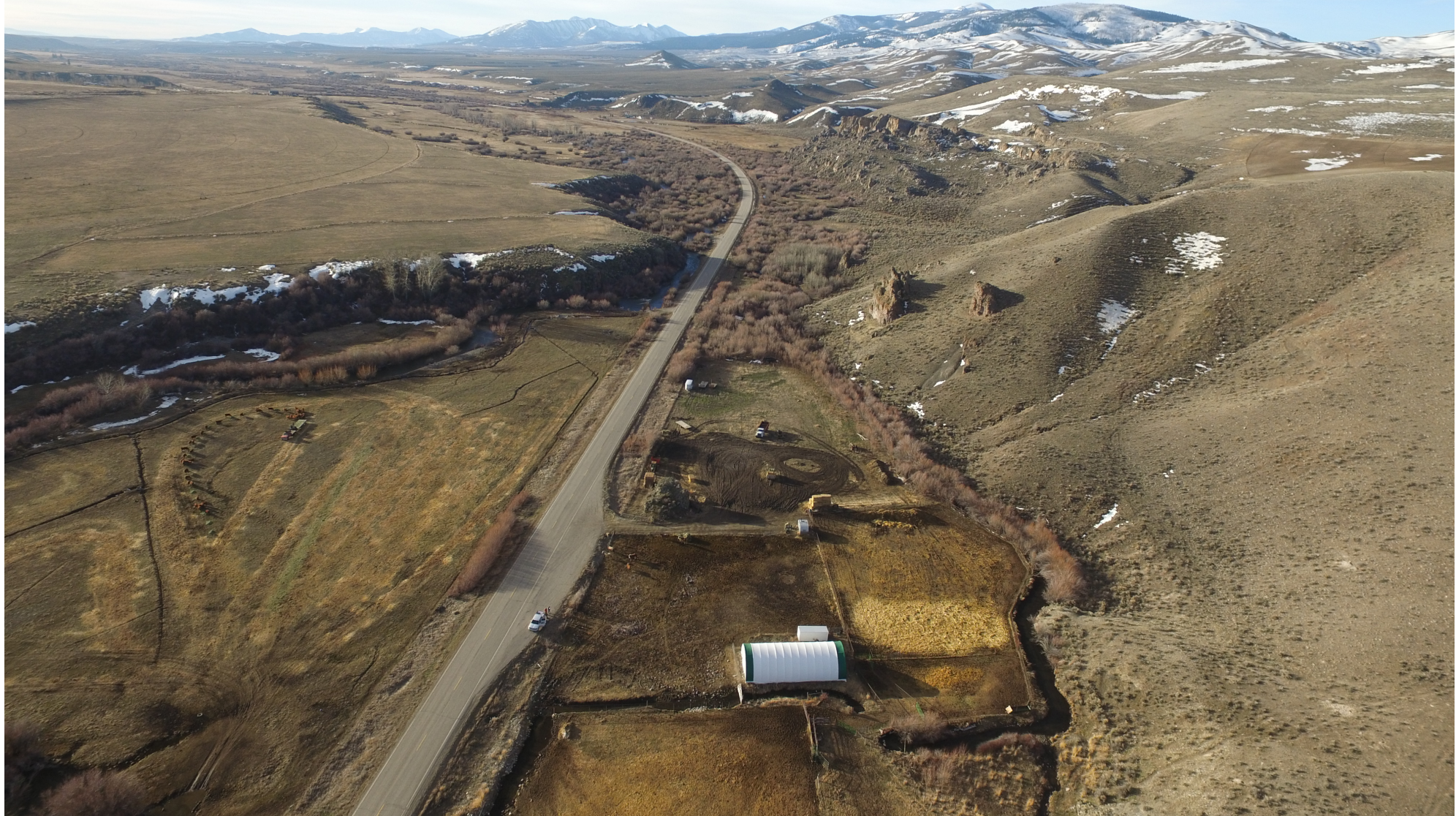
Aerial view of the project area as construction on new stream channel begins.
