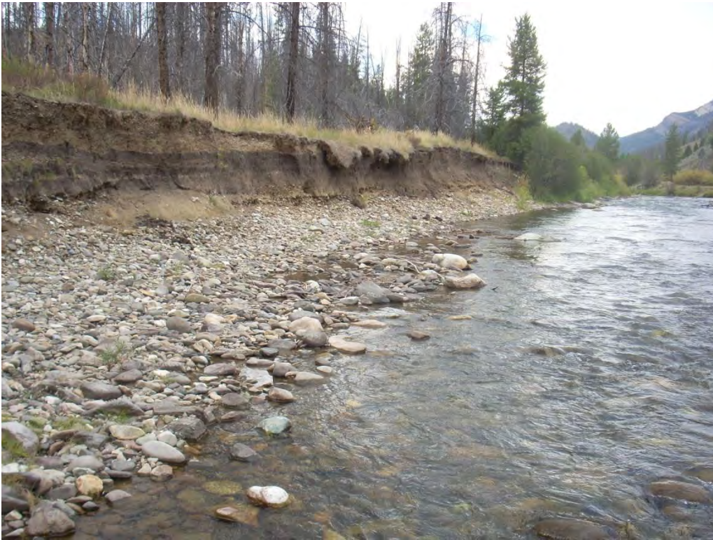
SO 84 – Unstable right bank, Reach 3, RM 6.3
