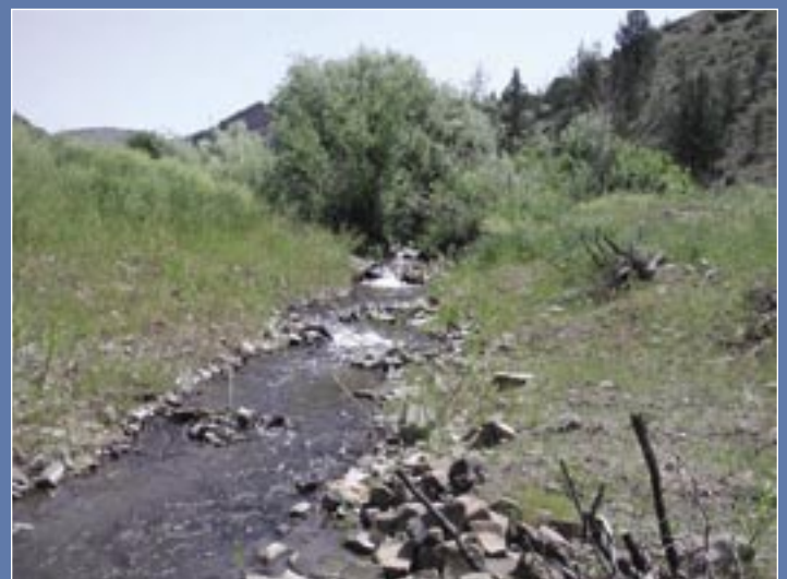
The same area after removing the culvert and rebuilding the creek channel.
