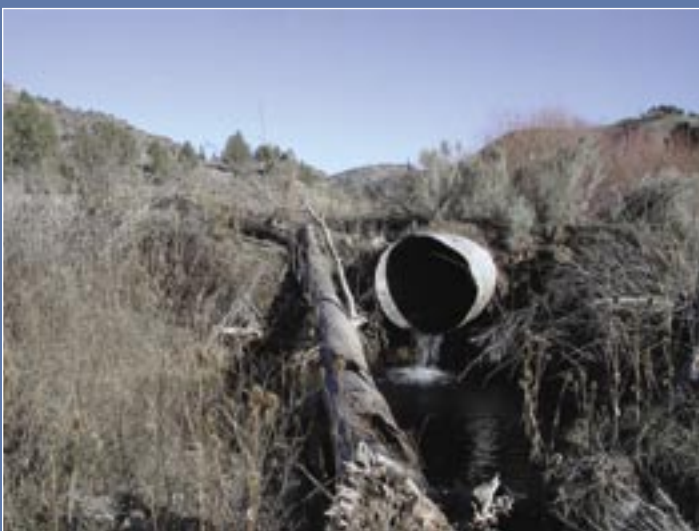
A Pine Creek culvert that was contributing to erosion.
