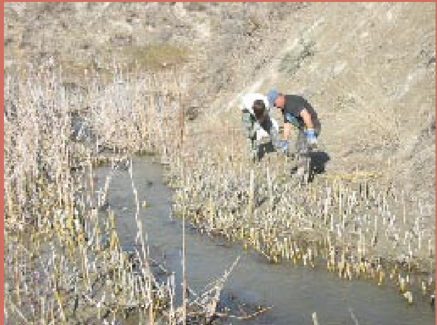
Planting willows along the shore of West Foster Creek will provide shade as the trees grow and reduce the water temperature, which is good for fish, and also provide forage and cover for wildlife.
