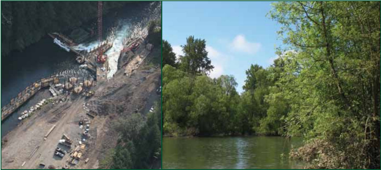
Left, the Minto fish-collection facility is being rebuilt downstream of Detroit Dam to improve the collecting, holding, sorting, and transportation of spring Chinook salmon and steelhead in the North Santiam River. Right, areas of fish habitat are being reconnected along the mainstem of the Willamette River, here in the Harkins Lake area east of Monroe. Photos: U.S. Army Corps of Engineers, left, and the Greenbelt Land Trust, right.
