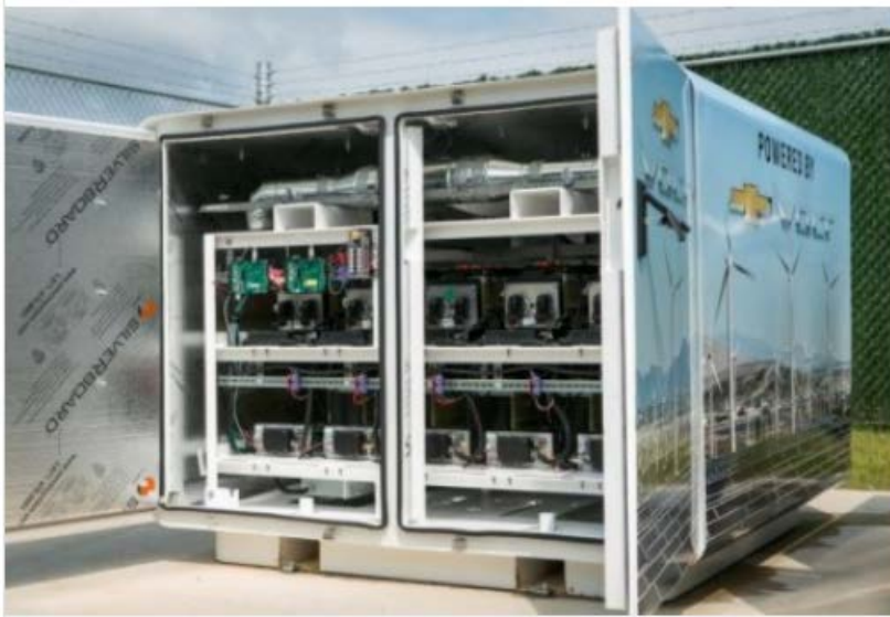
Used Chevrolet Volt batteries are helping keep the lights on at the new General Motors Enterprise Data Center at its Milford Proving Ground in Milford, Michigan. Five Volt batteries work with an adjacent solar array and two wind turbines to help supply power to the data center's administrative offices. (Photo by John F. Martin for General Motors)
